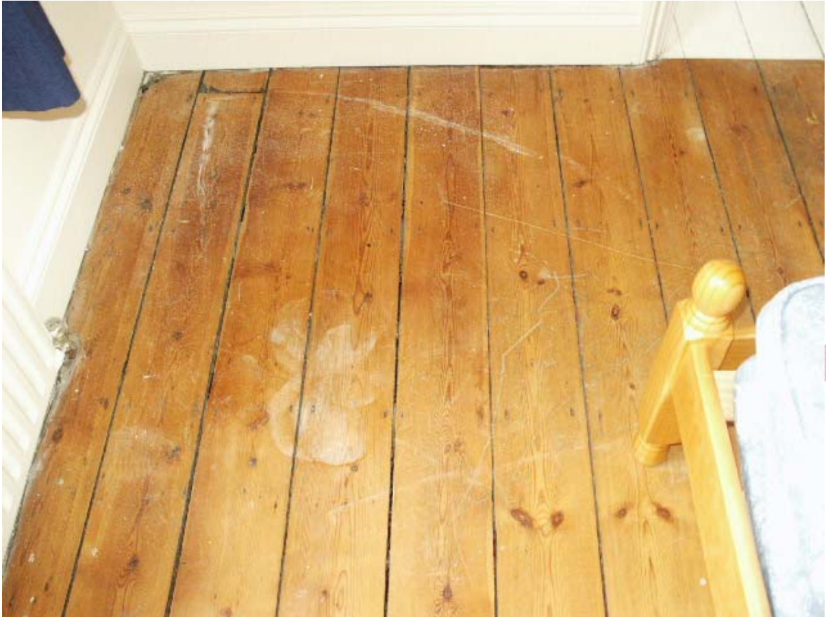
Bedroom 4 – scratches and marks to floor
