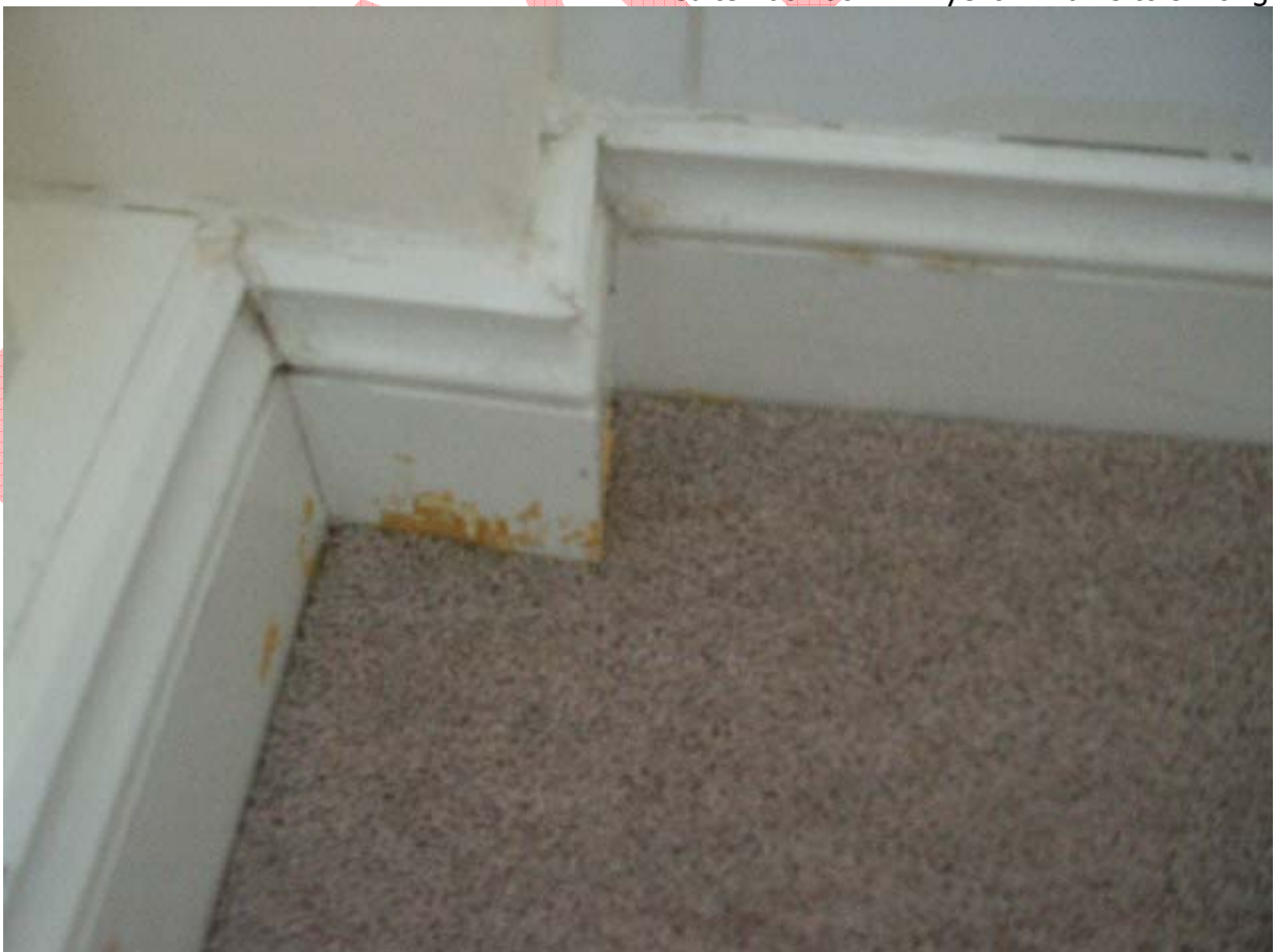
En-suite Bathroom 2 – yellow marks to skirting
