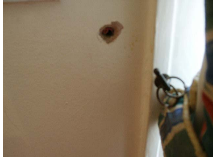
kitchen – hole in wall behind curtain
