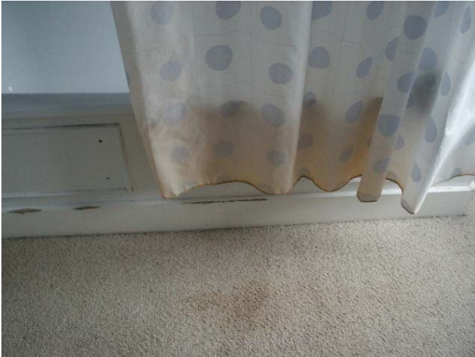
Bathroom – stains to carpet & shower curtain
