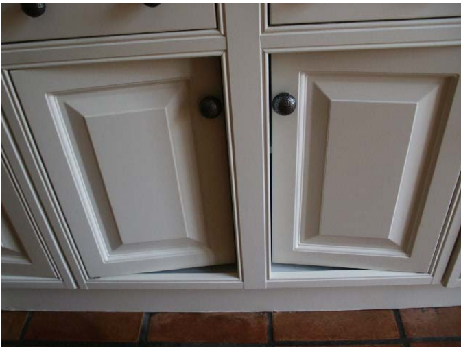
Kitchen – doors do not shut
