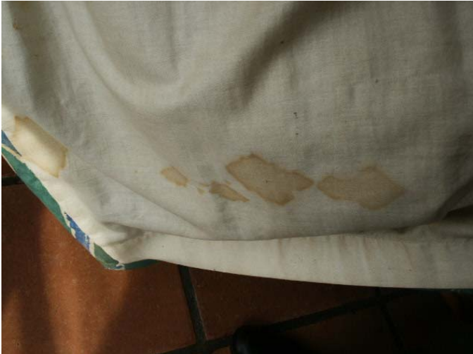
Kitchen - water marks to curtain
