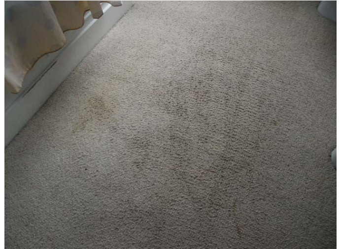
Bathroom – stains to carpet
