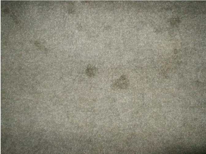
Reception Room – spots & stains to carpet
