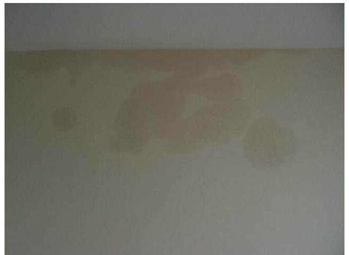
Bedroom 5 – damp marks to wall
